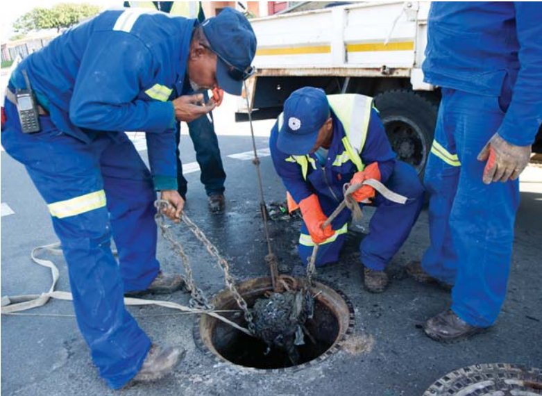
Dirty work: Clearing sewerage blockages caused by dumping costs R270 million a year.
