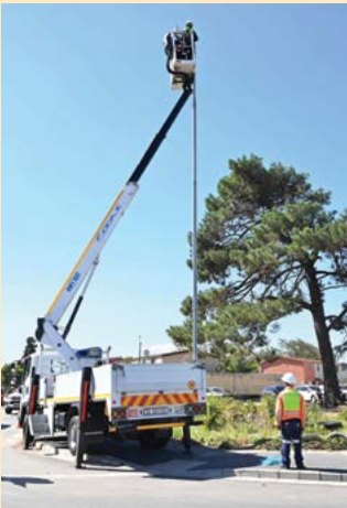
Help us shine a light on vandalism: The City calls on residents in streetlight vandalism hotspots such as Scottsdene in Kraaifontein to report suspicious behaviour relating to public lighting infrastructure.
