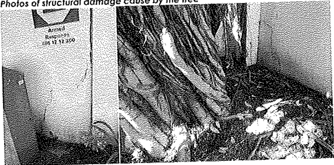
Photos of structural damage cause by the tree
