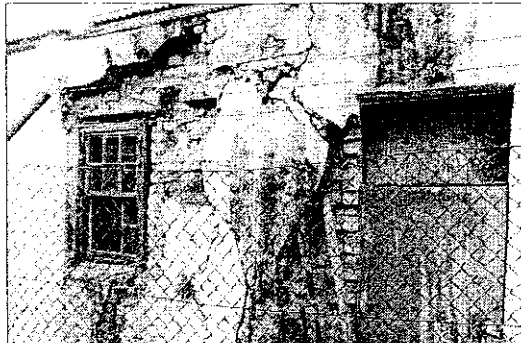
Run down and neglected, the old post office on Constantia Main Road.
