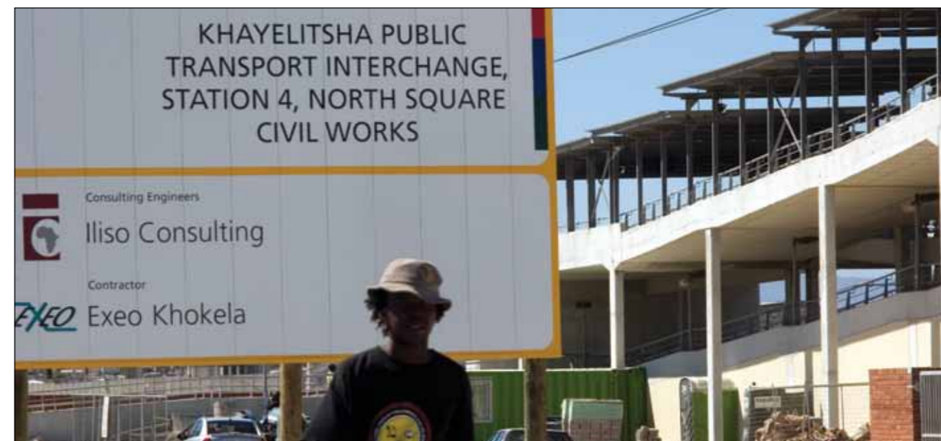
Upgrading and renovating, stations, roads and pavements has been an important part of the URP.
