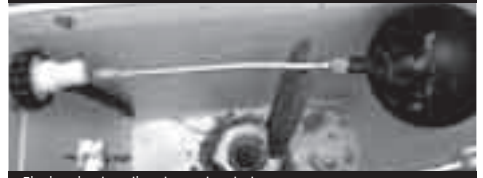
Flush valve in toilet cistern is missing
