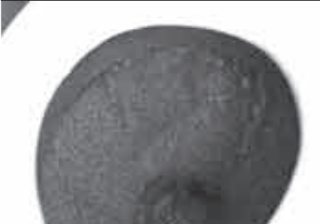
Leak into toilet bowl
