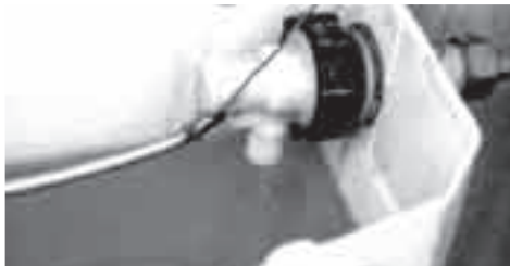
Toilet cistern float valve leaking
