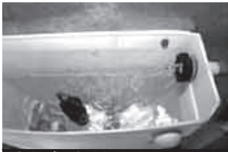
Toilet cistern float valve missing
