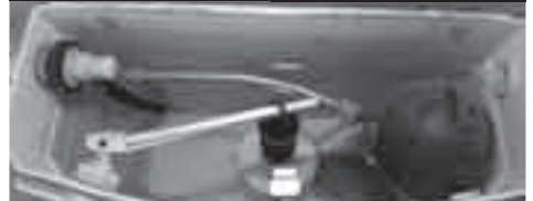
Toilet cistern has buckled because the lid has been left off
