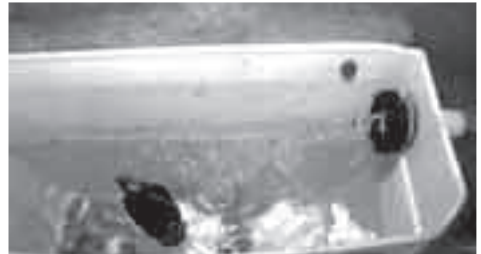
Toilet cistern float valve missing
