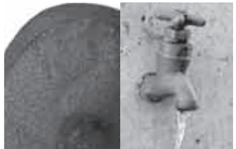
Leak into toilet bowl
