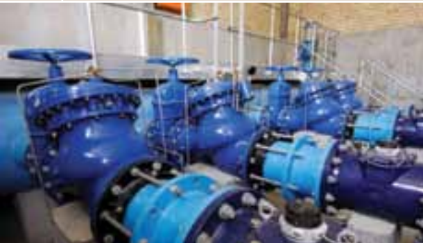
Mitchells Plain pressure management installation
