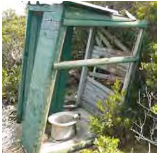
The abandoned and derelict ablution at Klippies Bay that should be demolished.
