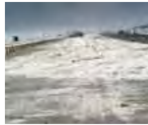
Poor planning has resulted in the parking area at Cemetery Beach suffering from wind-blown sand problems, as it was built in a dynamic dune system. Cemetery Beach requires frequent and ongoing maintenance.
