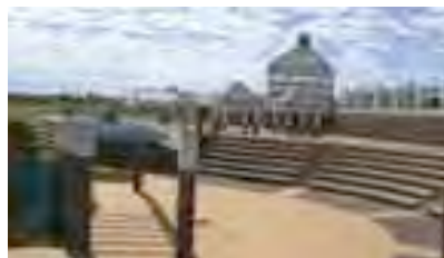
The Silwerstroom Strand Pavilion requires general maintenance work to bring it up to an acceptable standard.
