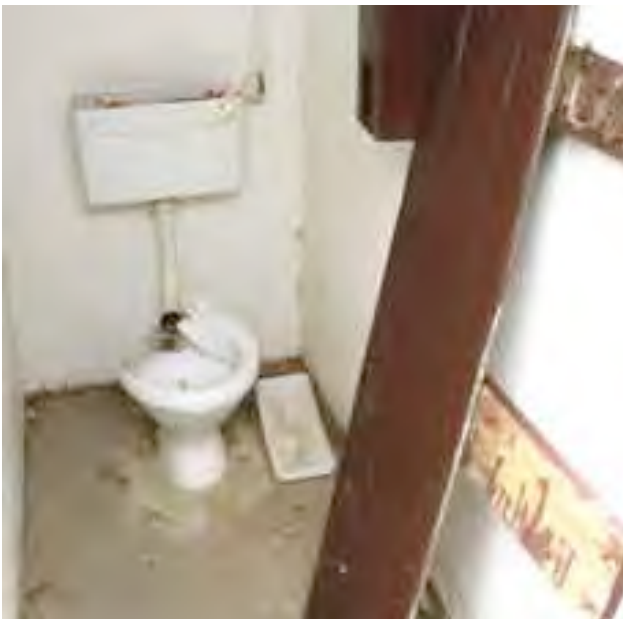
Broken and useless toilet at Klippies Bay.
